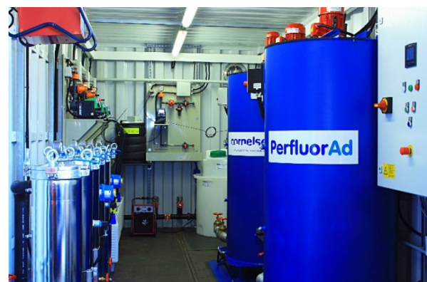
Figure 5: Mobile PerfluorAd treatment plant for the treatment of rinse water or extinguishing water
